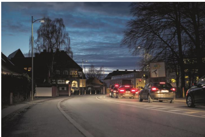
A truly connected solution for smart, energy efficient lighting in Copenhagen delivered by Thorn Lighting
