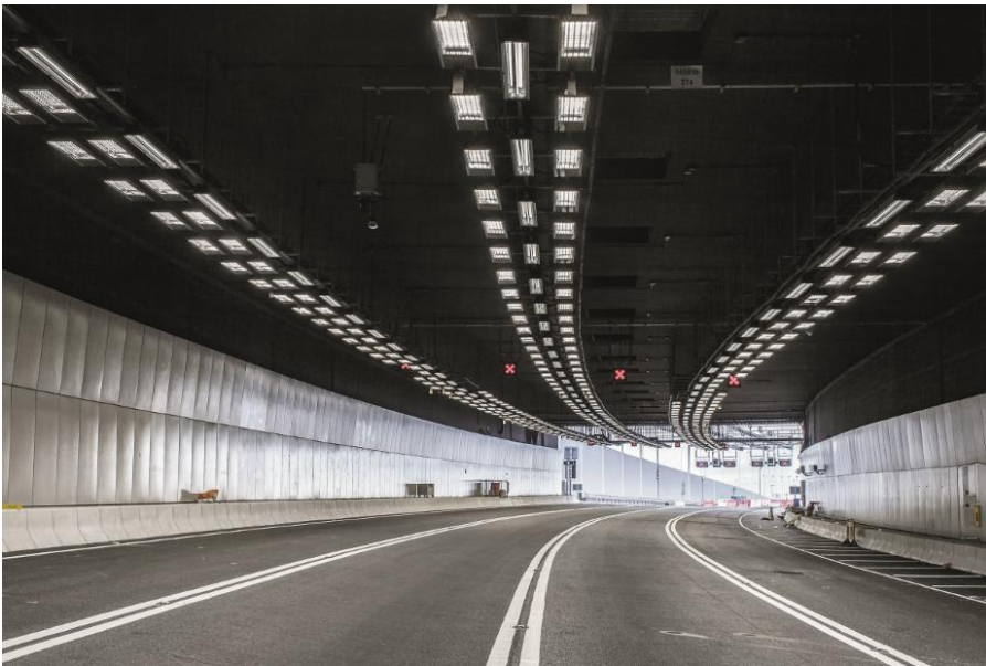
6000 of Thorn's GTLED Entry and GT58 luminaires with DALI drivers illuminate the one-kilometre tunnel.
