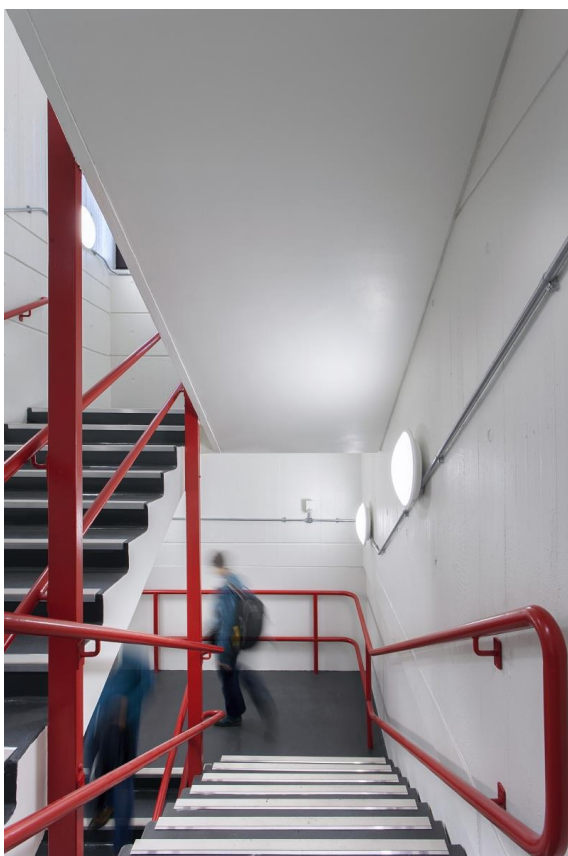
Image 2: Thorn's Novaline ensures that the right lighting levels are met for a safe stairwell illumination.
